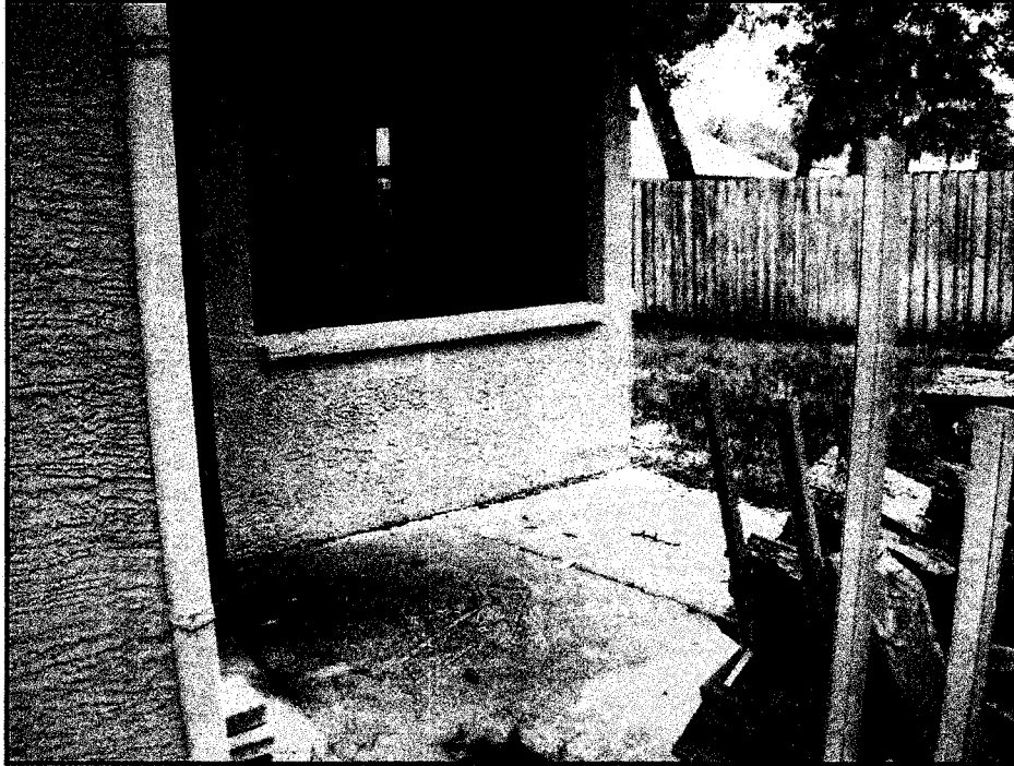
Photograph 27: A crack in concrete patio slab. (C)
