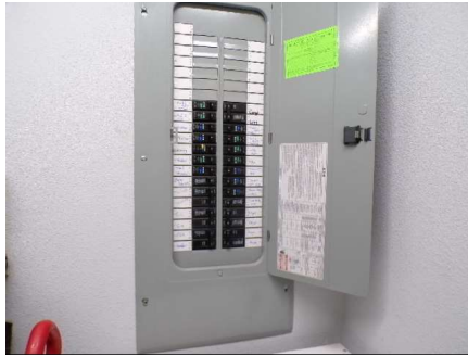
Main Electrical Panel
