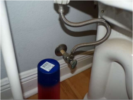
Bathroom Toilet Supply Valve
