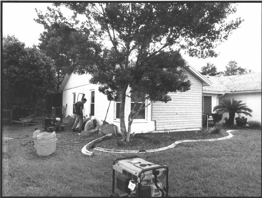
Photo 2: View of Pin installation along the targeted repaired area of the house.
