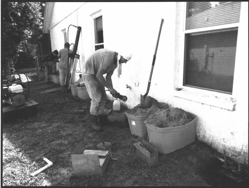
Photo 3: View of Pin installation along the targeted repaired area of the house
