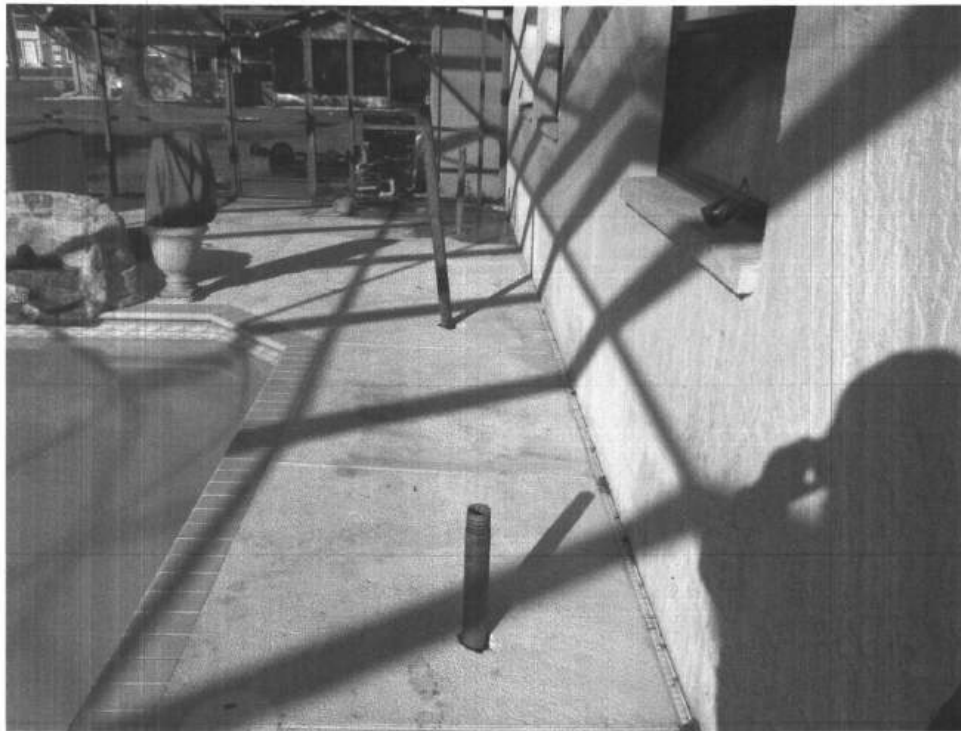
Picture 5: Core holes in pool deck
