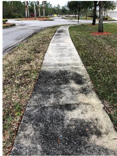
Example of Non-Compliant Sidewalk
