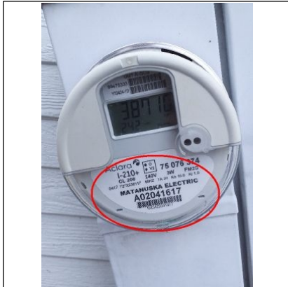
Photo of the electric meter located on the back of the home.
