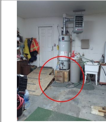
There should be a Bollard installed in front of the water heater in the garage for protection from possible vehicle impact.
