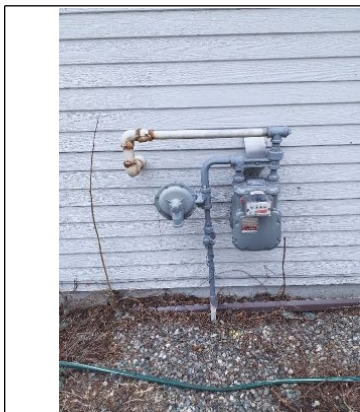
Photo of the gas meter located on the back right hand corner of the home.
