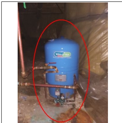
Photo of the well pressure tank located in the crawl space.
