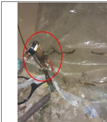
Photo of the main water shut-off valve located in the crawl space in front of the well pressure tank.
