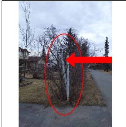
Recommend replacing the two exterior electrical outlets located on the two light poles on either side of the driveway with GFCI protected Outlets and the Light Pole located on the right hand side of the driveway needs to be restraighted its leaning in towards the home which could cause a problem with the electrical wiring.
