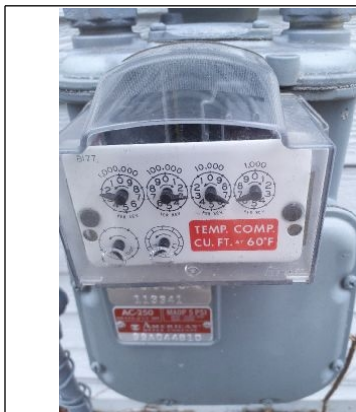
Photo of the gauges on the gas meter.
