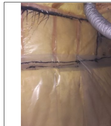
Photo example of the fiberglass insulation located on the Foundation walls in the crawl space.
