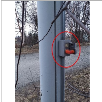
Recommend replacing the two exterior electrical outlets located on the two light poles on either side of the driveway with GFCI protected Outlets and the Light Pole located on the right hand side of the driveway needs to be restraighted its leaning in towards the home which could cause a problem with the electrical wiring.
