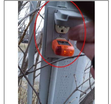
Recommend replacing the two exterior electrical outlets located on the two light poles on either side of the driveway with GFCI protected Outlets and the Light Pole located on the right hand side of the driveway needs to be restraighted its leaning in towards the home which could cause a problem with the electrical wiring.
