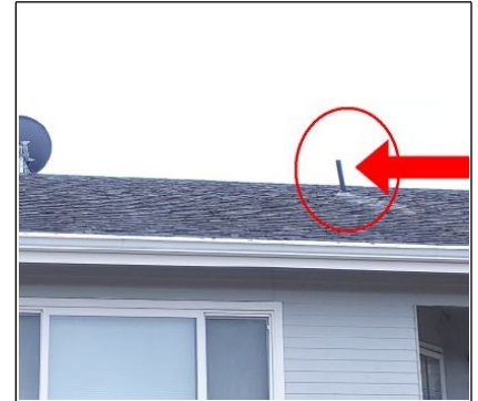
Recommend evaluation by licensed plumber for the repair of the plumbing vent located on the back side of the roof the right hand side of the satellite dish at the time the inspection you can see that the Plumbing vent is leaning to left hand side and it's no longer pointing straight up.
