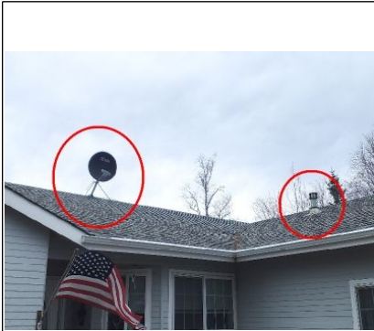
Photo of a satellite dish and flue for the gas space heater and water heater located in the garage.
