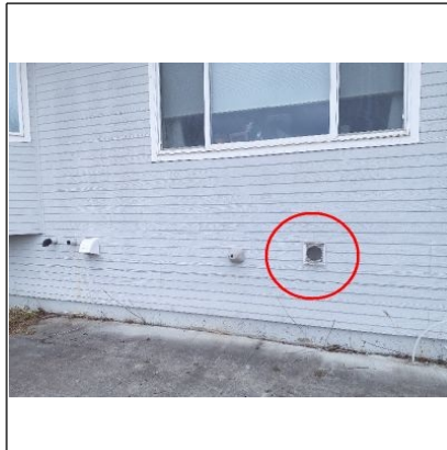
Recommend installing the missing vent cover for the exhaust vent located on the back of the home to the left hand side of the deck.
