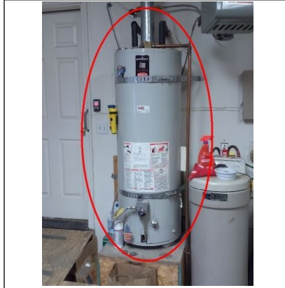
Photo of the water heater located in the garage.
