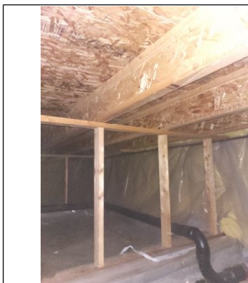
Photo example of the fiberglass insulation located on the Foundation walls in the crawl space.
