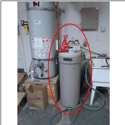
Photo of the water softening system located in the garage.
