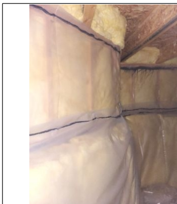
Photo example of the fiberglass insulation located on the Foundation walls in the crawl space.
