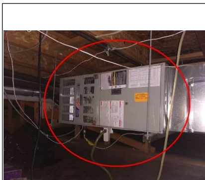
Photo of the Furnace located in the crawl space.
