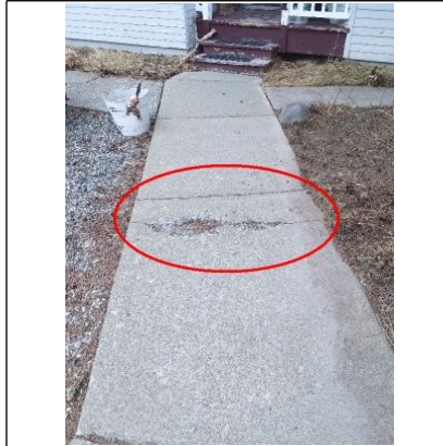
Recommend evaluation for repair of the deteriorating Concrete service walk leading from the garage to the porch located on the front of the home.
