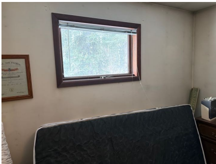
Back bedroom - over 48" from the floor
