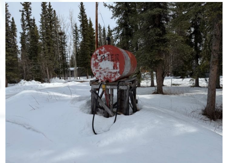
Vehicle fill tank
