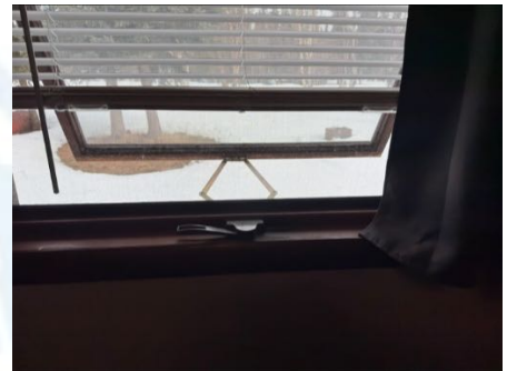
Second front bedroom - wrong hardware
