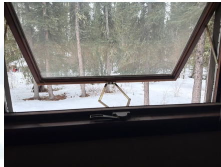
Back bedroom - wrong hardware/too small
