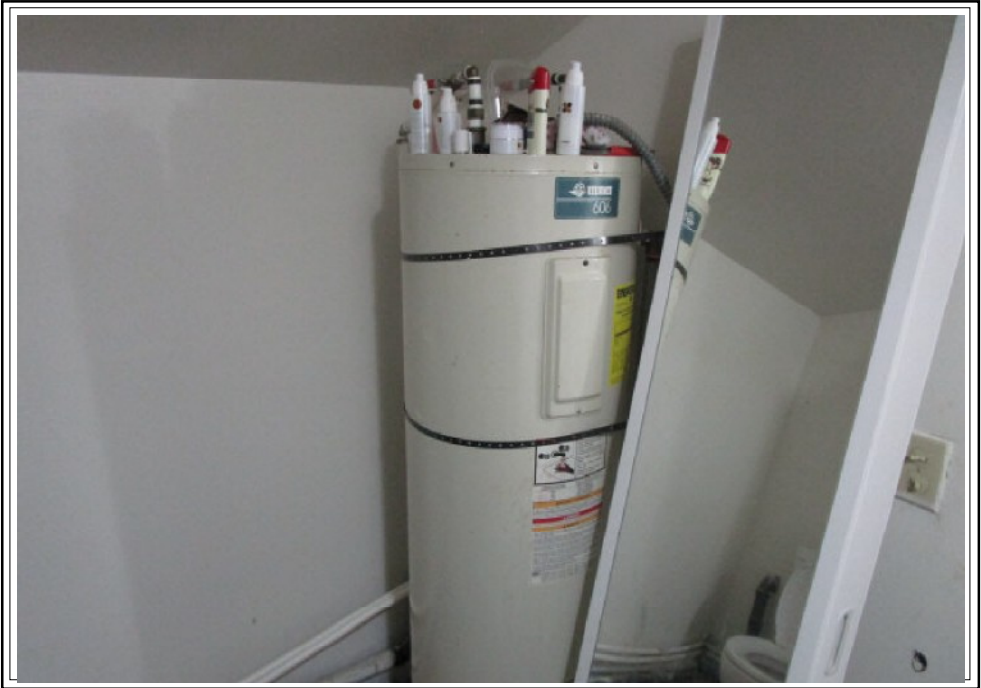
Hot water heater has both straps.
